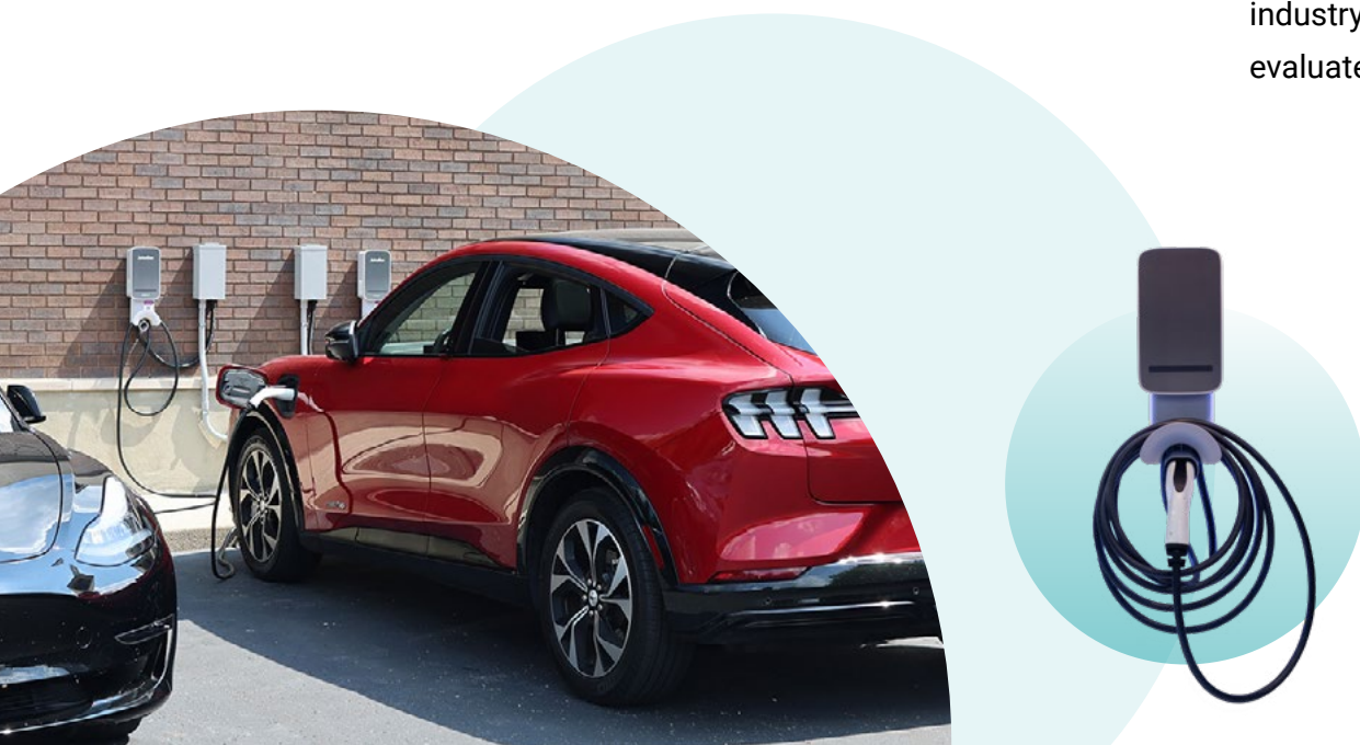
EV Charging Stations at HQ
